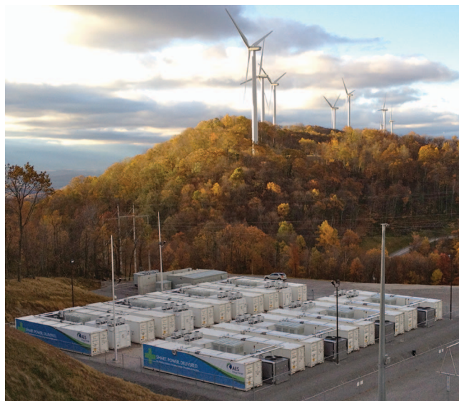
Figure 2. A 32 MW LiFePO 4 battery at a wind power farm in West Virginia. (Photo courtesy of AES Energy Storage.)
